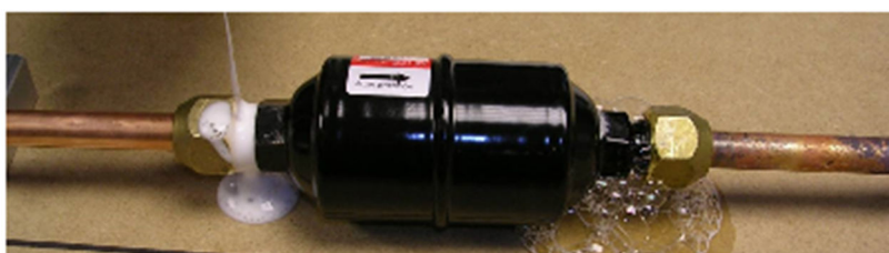
example of bubbling caused by leakage
